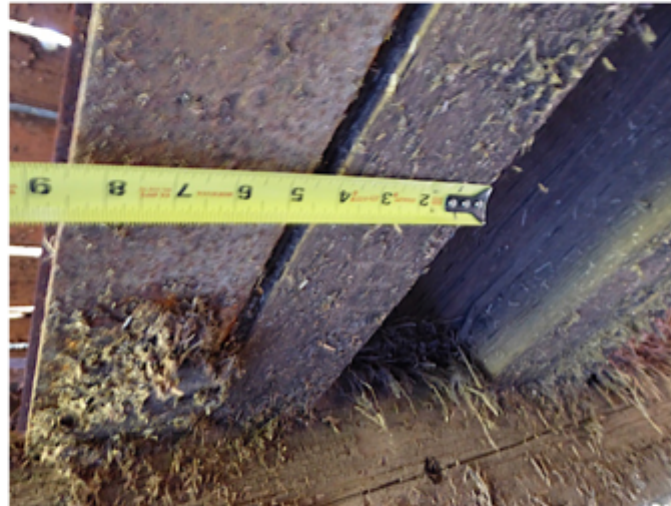
i-beams are about 4" wide and the i-beam + wood timber are about 8.5" wide.
