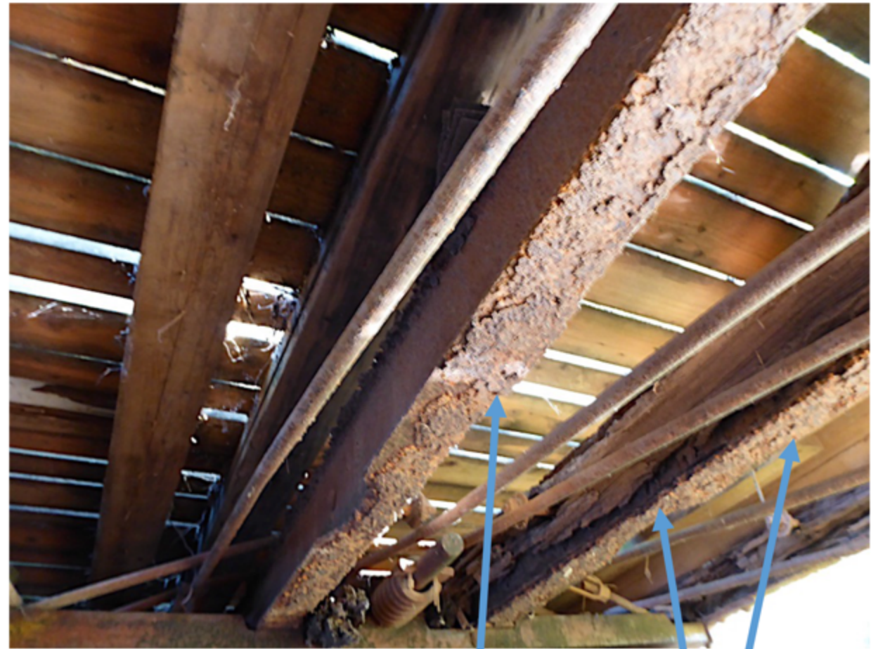
Eastern Bridge: I-beams Rusted through at edges and wood beams gone or nearly gone.
