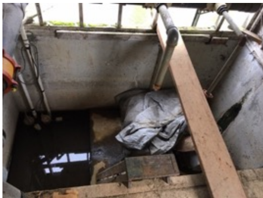
Pumps under tarps below waterline
